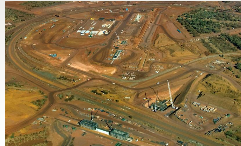
Above: Construction of Jimblebar, including new rail loadout, May 2008 Below: Construction of the Newman Hub, May 2008
